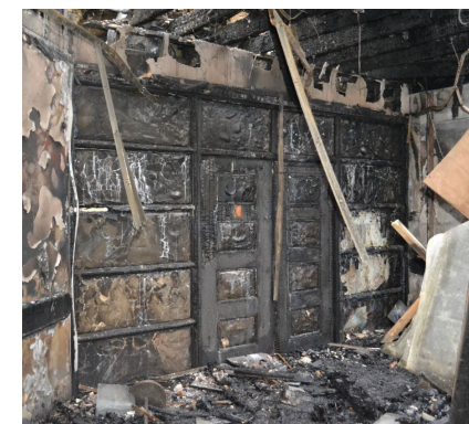
Internal side of fire door after fire
