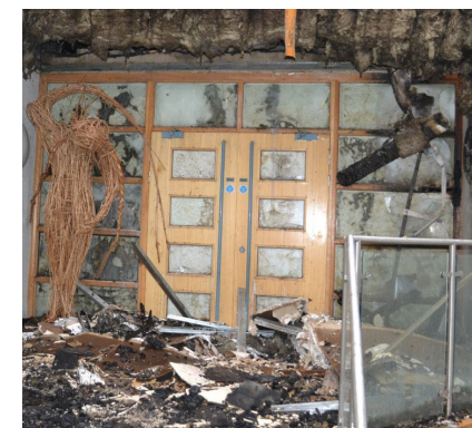
External side of fire door after fire
